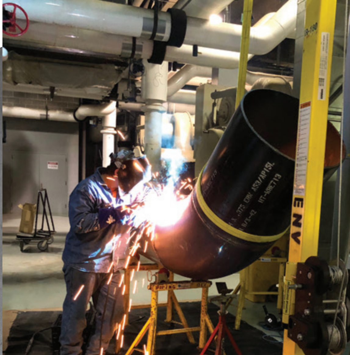
A 24" river water piping being fabricated for a chilled water plant in the Loop.
